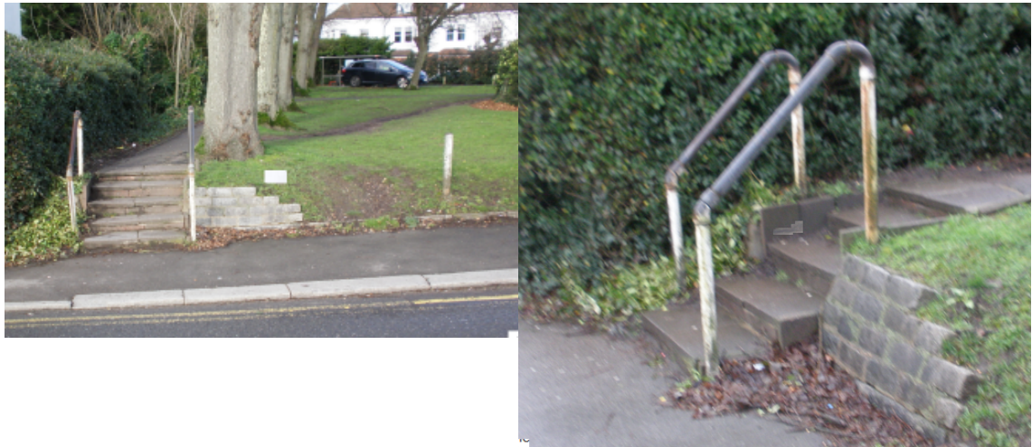
Fig 2.3 – Worn Grass Area and Poor Standard Steps
